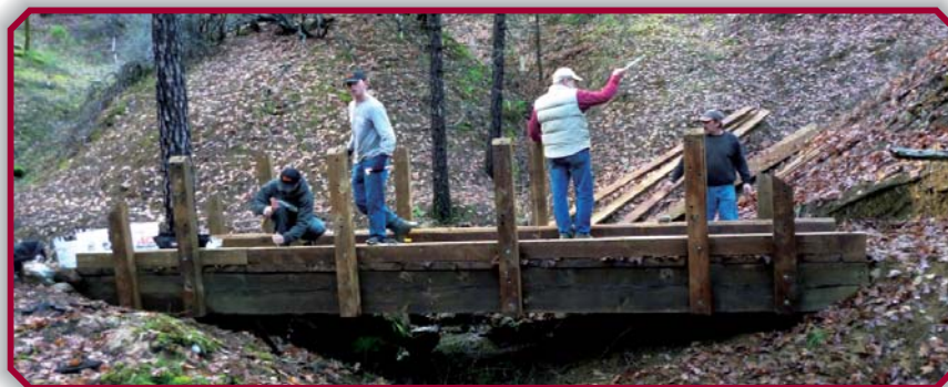
Installation of handrails by TCRCO employees (l-r) Jeff McGrew, Duke Klang, John Condon and Darrel Tate. Doug Crispin works on underside of bridge.
