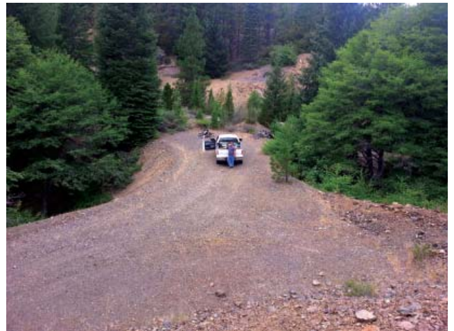
Before construction to remove 84" culvert and reconstruct this section of the West Fork of Hayfork Creek.
