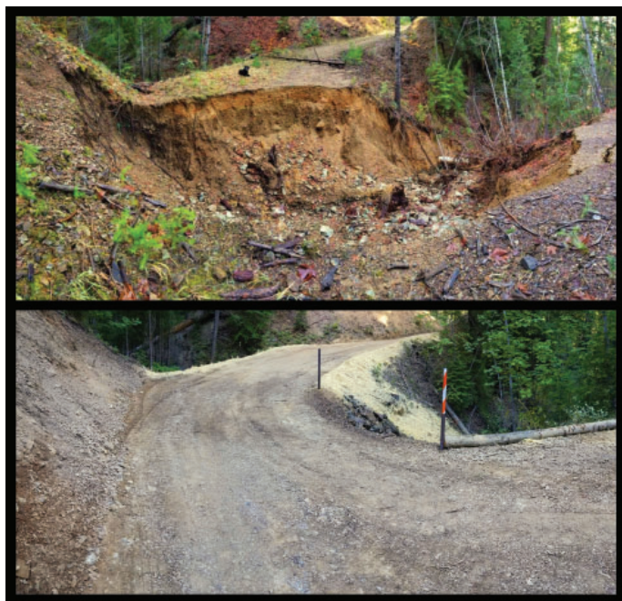
Washed out stream crossing repair due to plugged culvert at Rattlesnake Creek
