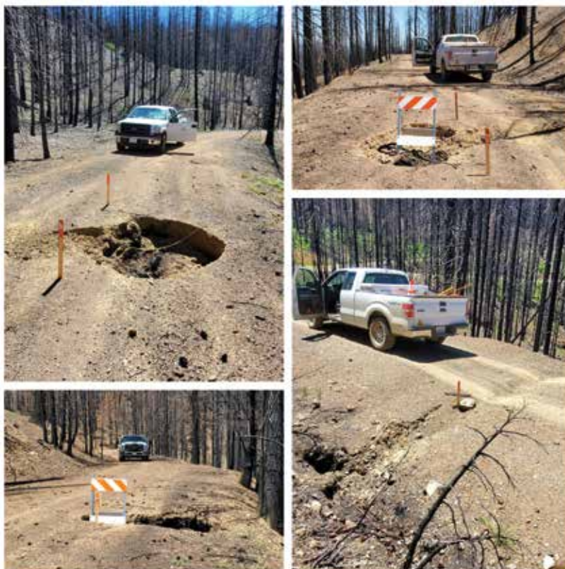
Following severe fire, roads often need extensive repairs.
