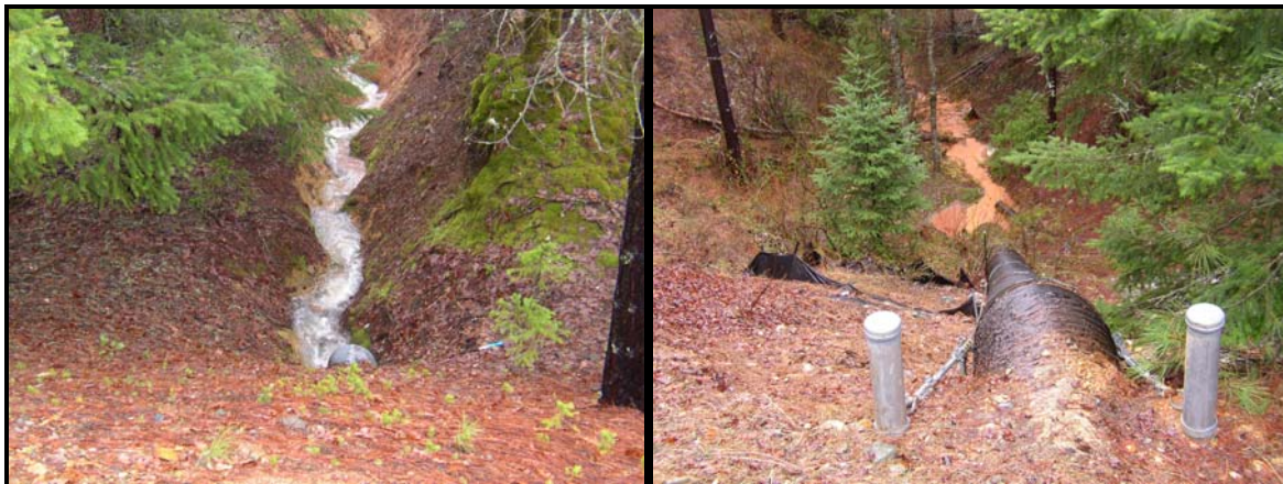
Photo 5-2 Outlets of culvert at mile marker 62.13 and 61.81 showing difference in turbidity levels.
