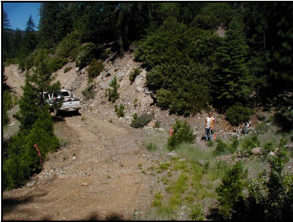
Photo 5-3. View of culvert with sediment filled inlet basin. Water has been flowing across road and downcutting road fill. Lack of minor maintenance could lead to crossing failure.
