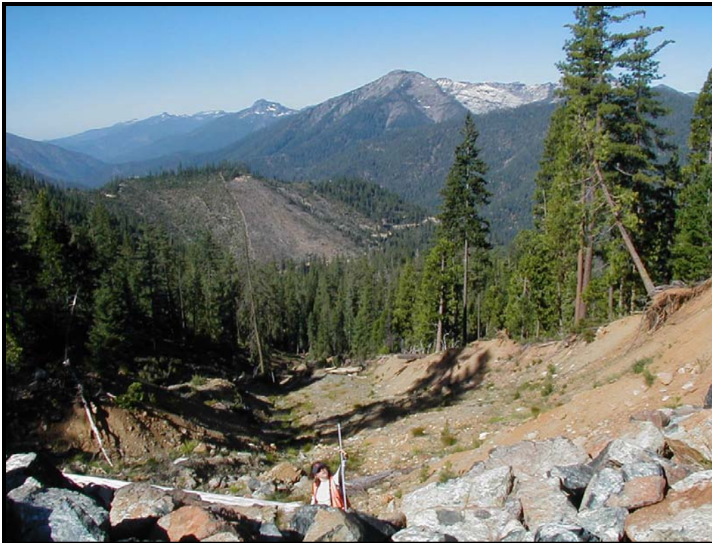
Photo 5-4 Measuring fill slope at culvert outlet. Riprap in foreground was placed to re-enforce road after landslide (mid-photo) event.
